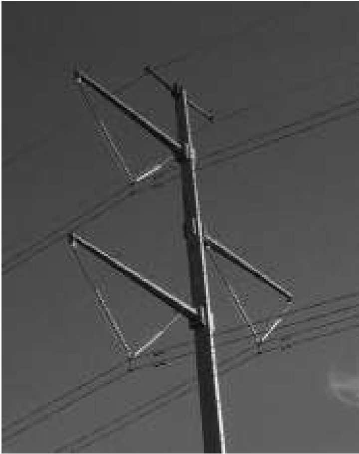
Figure 1.4a Steel Pole with V-String Insulators.
