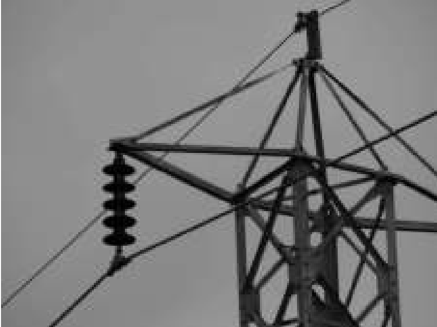
Figure 3.11 Insulator Attachment to Lattice Tower.
