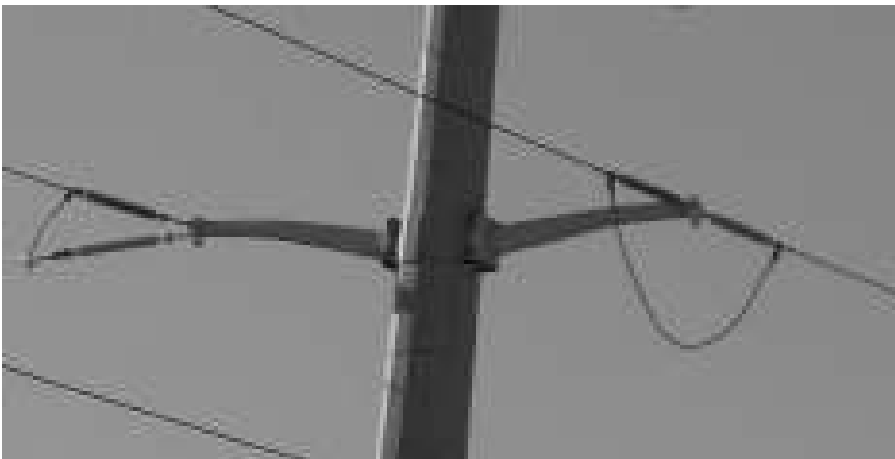
Figure 3.13 Insulator Attachment to Steel Pole.
