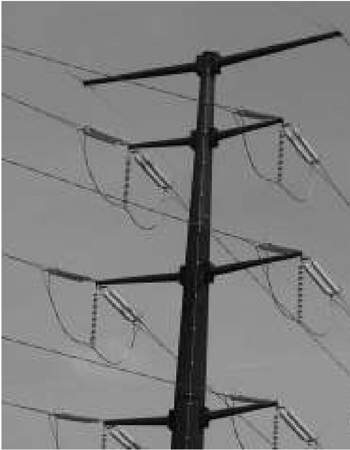
Figure 1.4c Steel Pole – Deadend Tangent.
