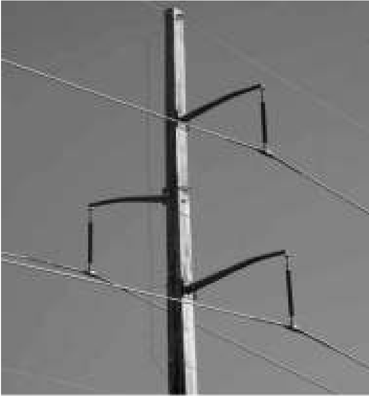
(c) Suspension Insulators on Steel Davit Arms
