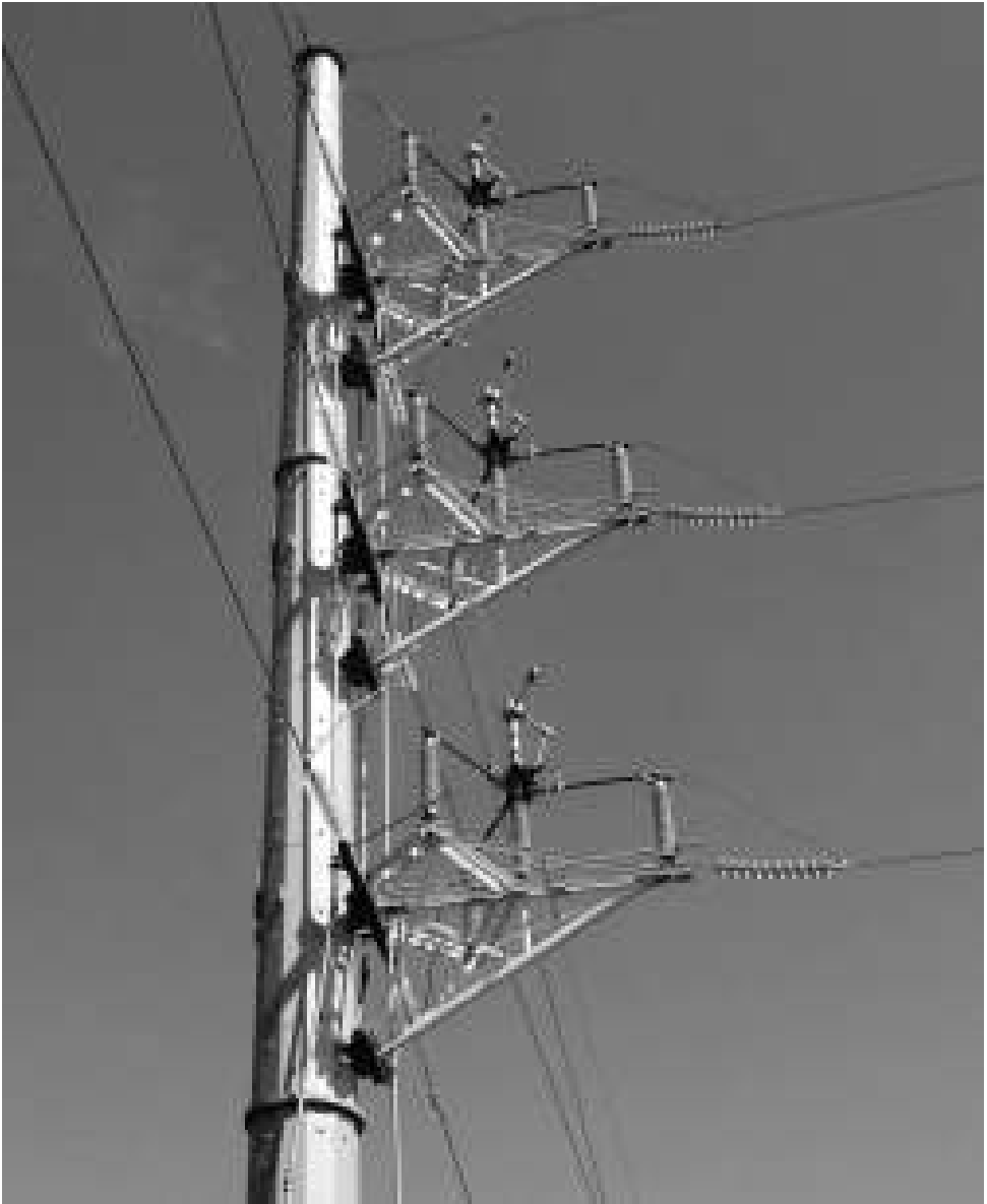
Figure 3.24 Air Break Switch.
