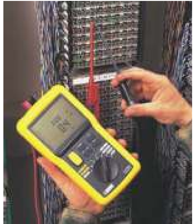
Figure 60: Insulation measurements on telephone cables
