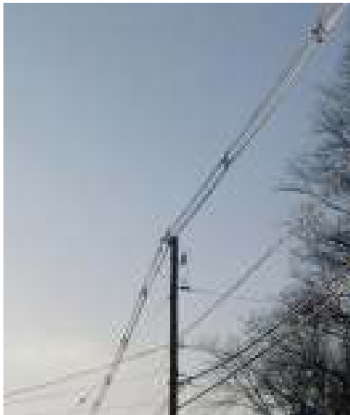
Figure 2.4 13.2-kV spacer cable.
