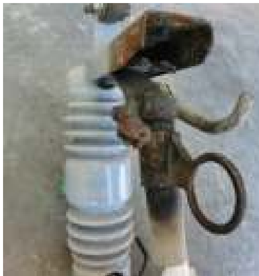
Figure 7.25 Cutout damaged by arcing in the field.
