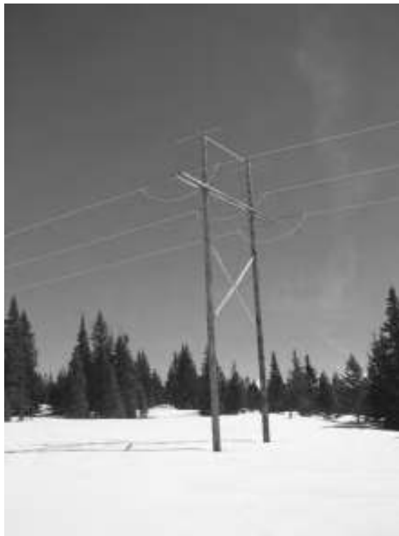
FIGURE 19.1 220 kV line with H-frame wooden towers.
