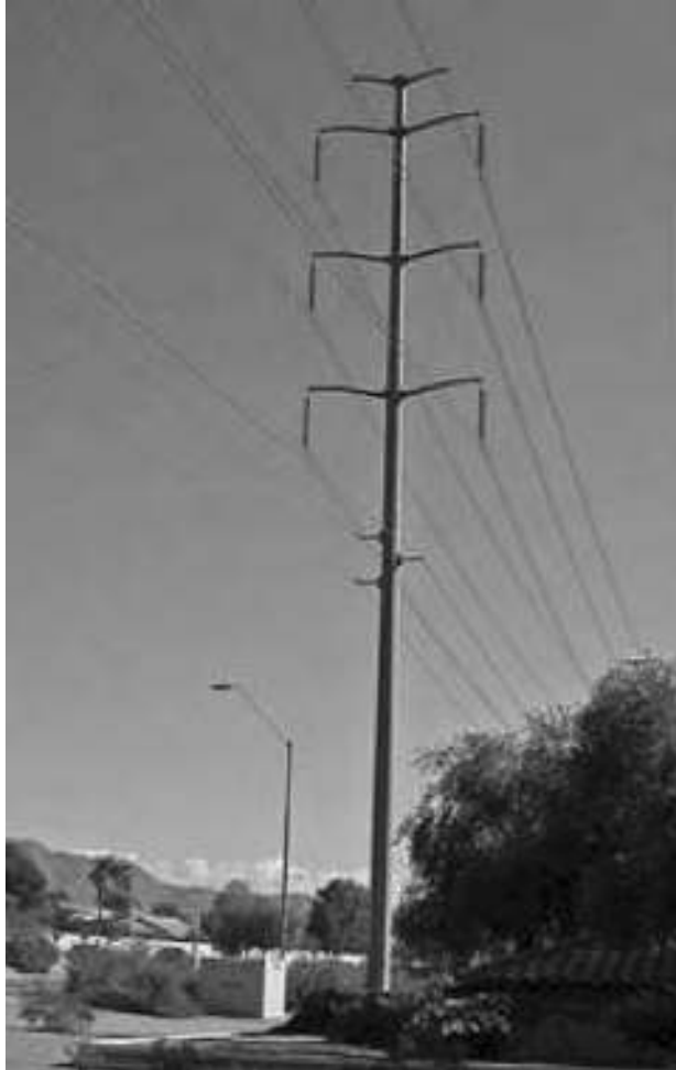
FIGURE 19.4 A 220 kV suspension tower.
