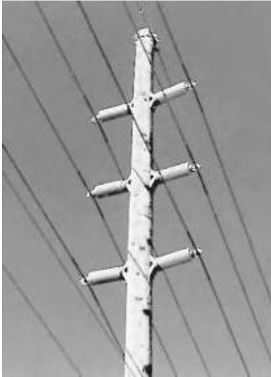
FIGURE 10.2 69-kV transmission line with post insulators.
