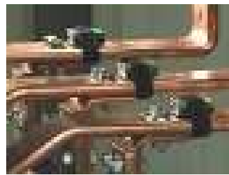
Figure 1.8. Set of Easergy TH110 sensors fixed on the 3 phases of an electrical connection
