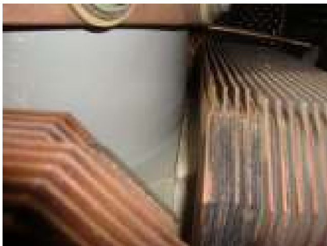
Figure 10.4 Contamination of a strip-on-edge field winding pole.
