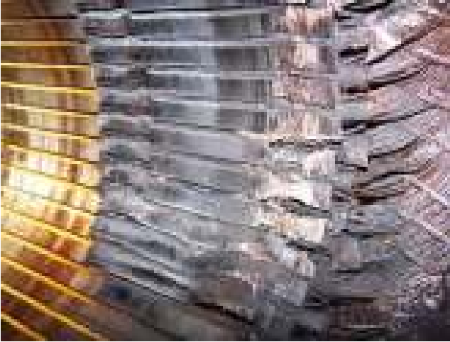
Figure 13.10 Stator rub on bore from bearing failure.
