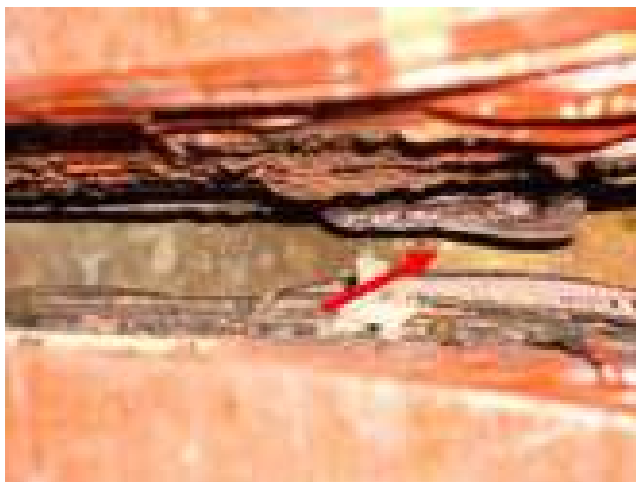
Figure 9.3 Failed pole jumper connection.
