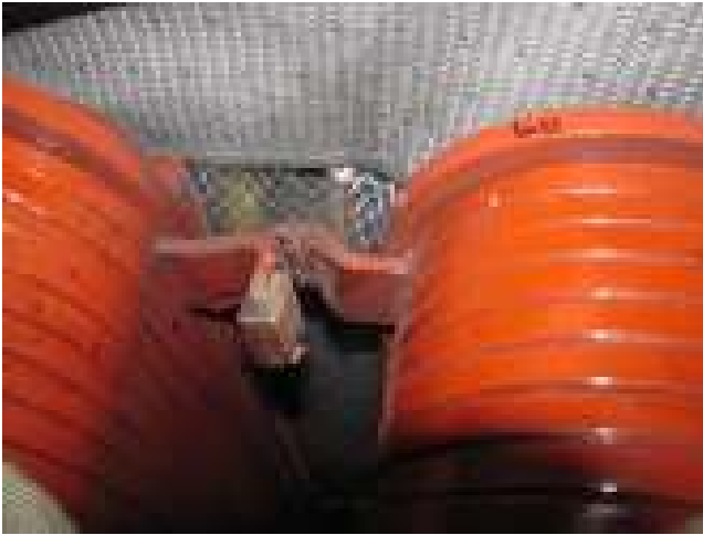
Figure 10.3 Failure of inter-pole connection from thermal cycling.
