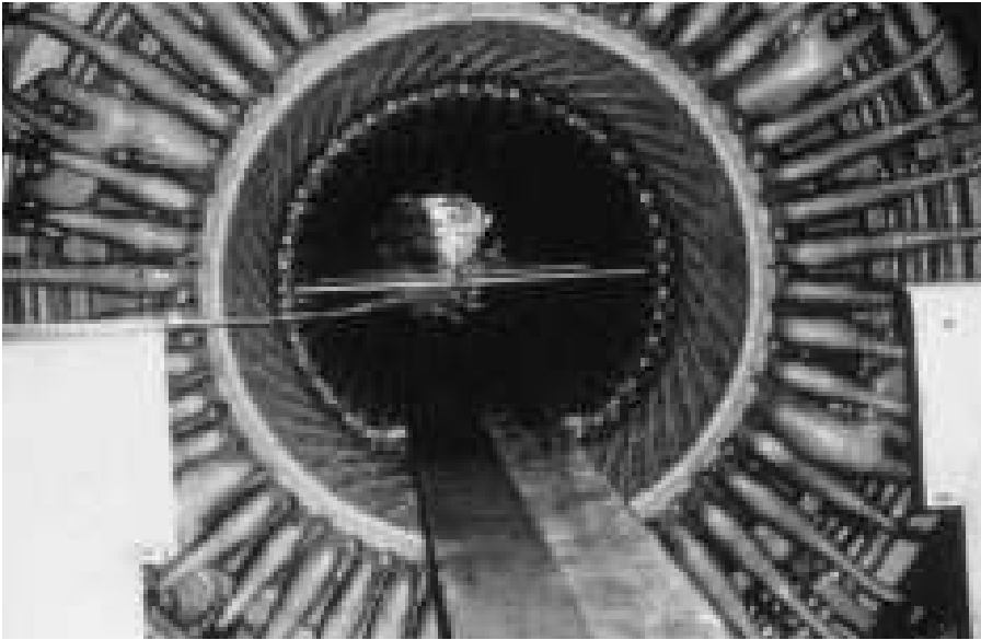
Figure 14.4. Photo of the excitation winding through the axis of a turbogenerator stator. (Courtesy Ontario Hydro.)
