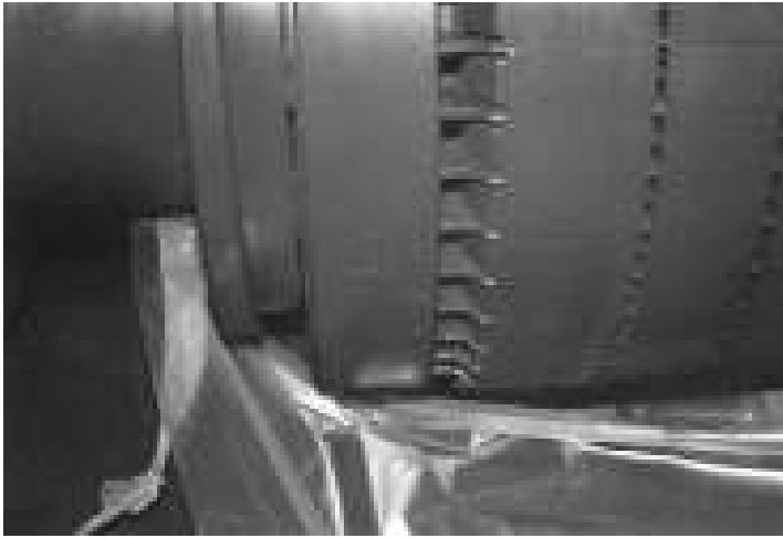
Figure 9.4. Photograph of a retaining ring over a short-circuit ring.
