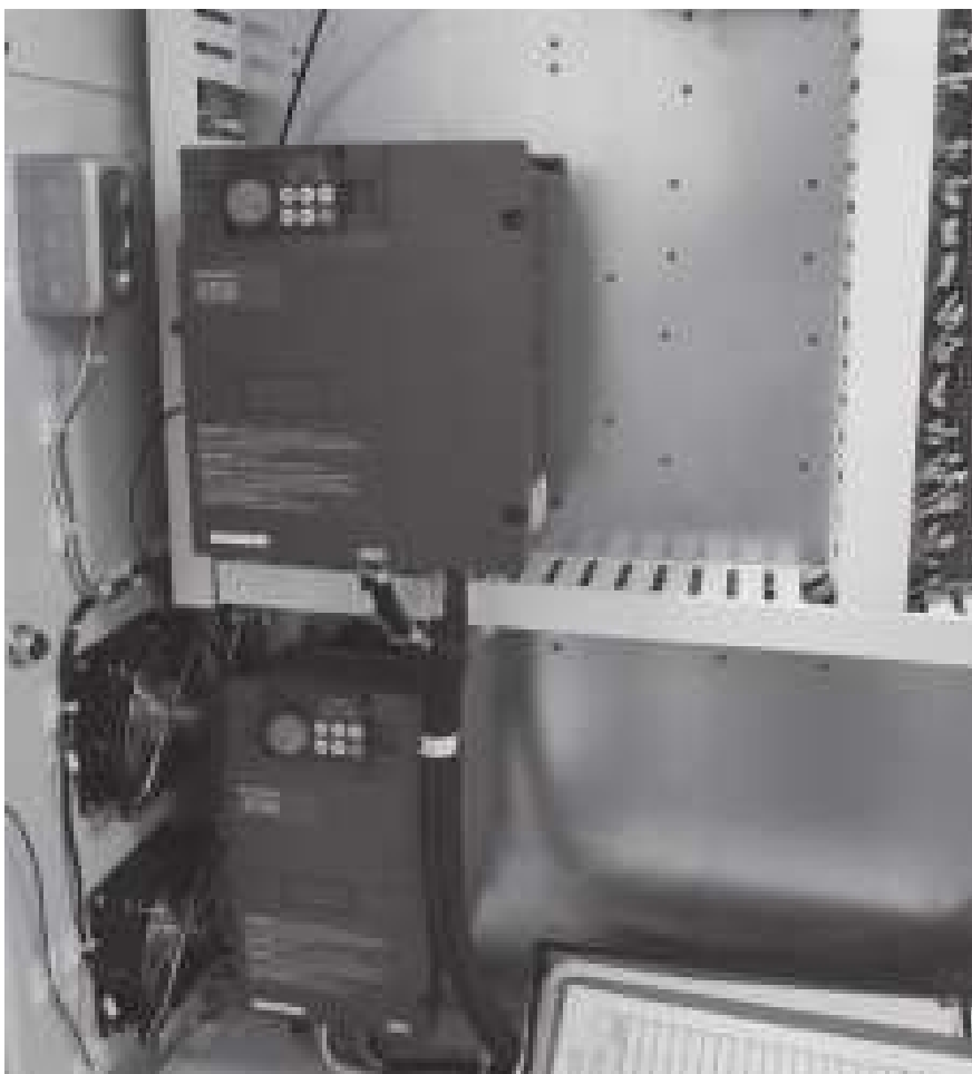
FIGURE 15-1 Solid-state motor controllers mounted in cabinets.
