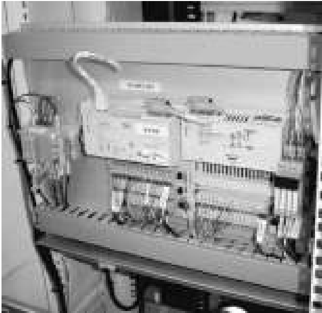
FIGURE 8.2 Example PLC installation.
