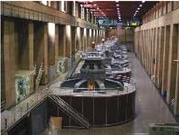
(b) Generating Hall: Hoover Dam
