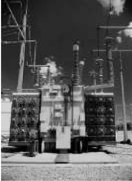
FIGURE 4.16 A large power transformer. Source: http://images.google.com/images?q=photos+of+power+transformers
