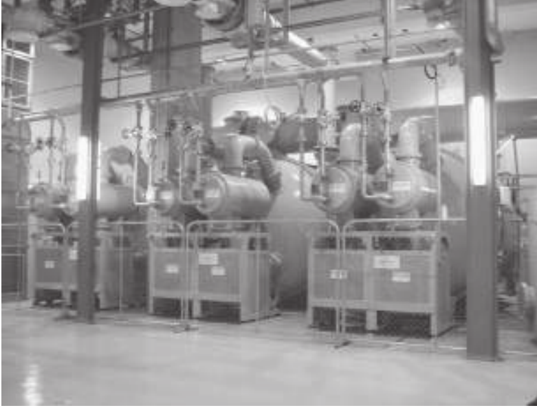
Haymarket substation (Australia)
