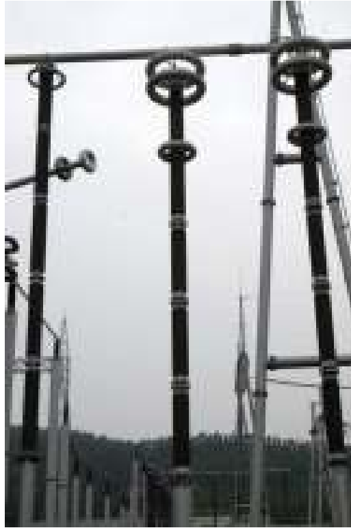
Figure 10.9 Surge arrester on Yunnan–Guangdong HVDC. Reproduced with permission of Siemens.
