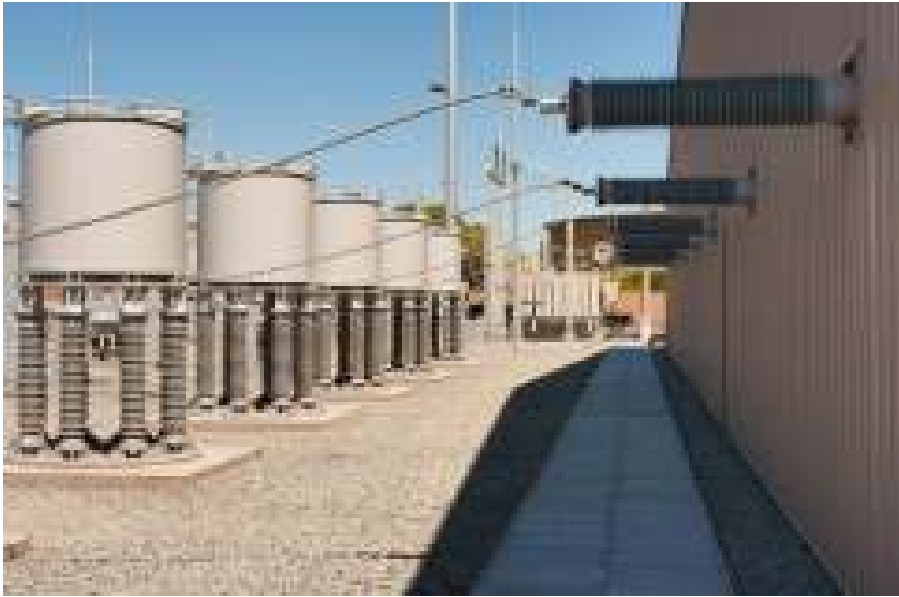
Figure 16.12 Arm reactors at Trans Bay MMC HVDC station. Reproduced with permission of Siemens.
