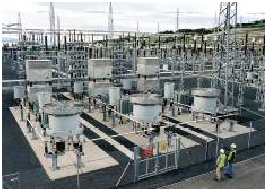
Figure 11.2 AC filters at Moyle HVDC station (2001). Reproduced with permission of Siemens.
