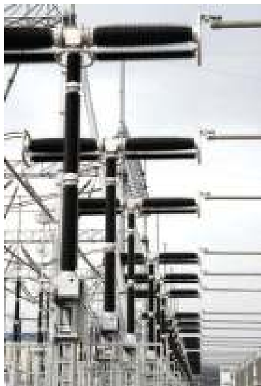
Figure 10.7 DC circuit breakers on the Yuannan–Guangdong HVDC. Reproduced with permission of Siemens.
