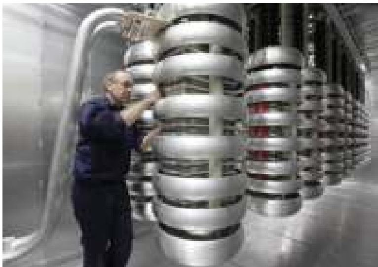
Figure 13.10 Testing VSC HVDC valves on BorWin1 project. Reproduced with permission of ABB.
