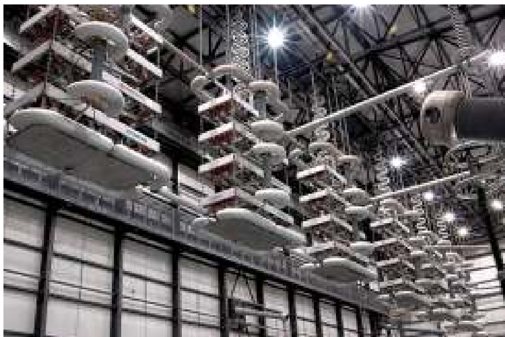
Figure 2.12 Thyristor valve hall at Yunnan-Guangdong HVDC station. Reproduced with permission of Siemens.
