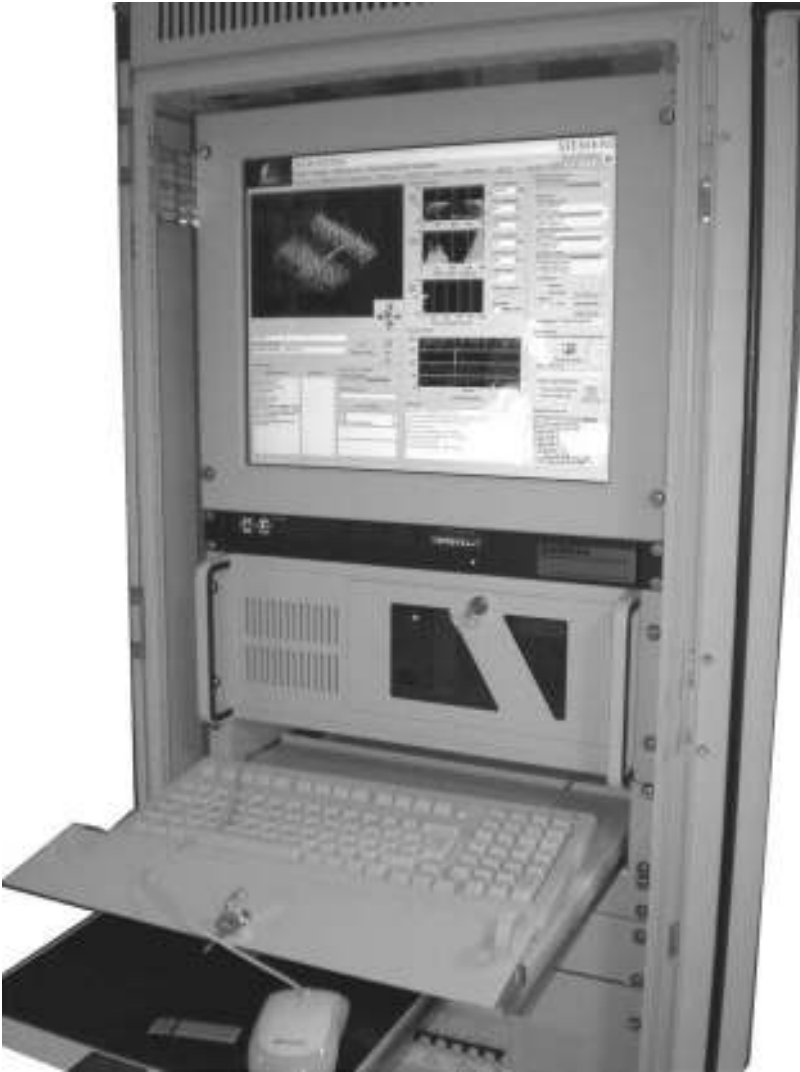
Figure 21.30 ISCM control cubicle showing PDM diagnostics display
