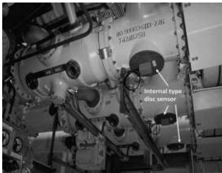
Figure 21.8 UHF sensors installed at Killingholme 420 kV GIS (1991)
