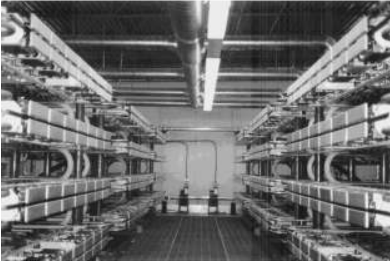
Figure 4.4 View of McNeill valve hall
