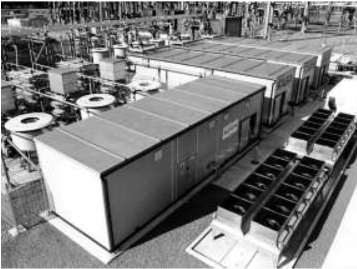
Figure 4.22 View of 225 MVA STATCOM
