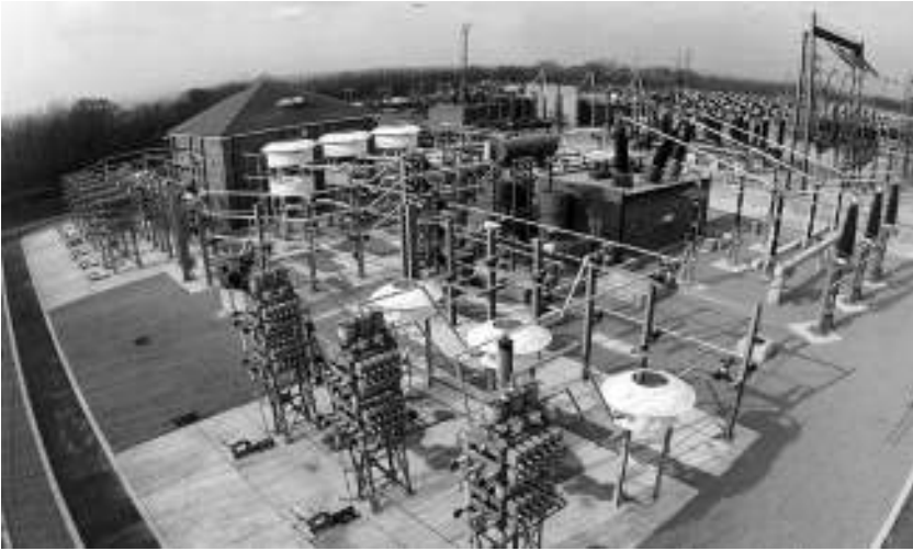
Figure 4.19 View of 225 MVA SVC
