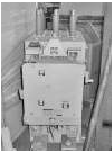
FIGURE 7.9 Vacuum circuit breakers
