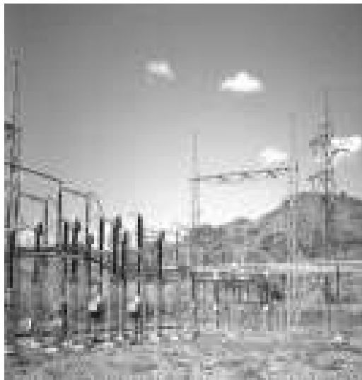
FIGURE 12.14 Switchyard using rigid bus-work
