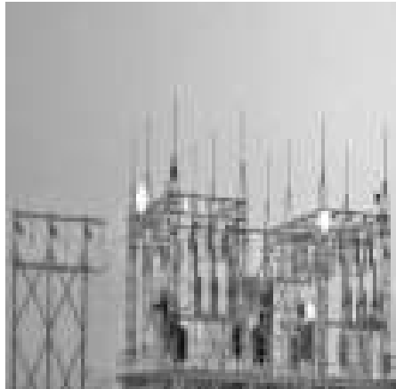
FIGURE 12.17 Switchyard protected by masts
