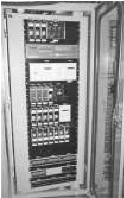
FIGURE 12.12 Swing-rack-type relay panel
