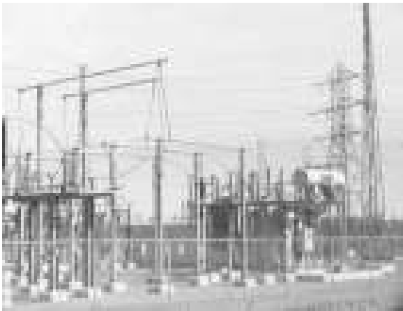
FIGURE 12.2 Typical outdoor low-level A-frame high-voltage transformer station
