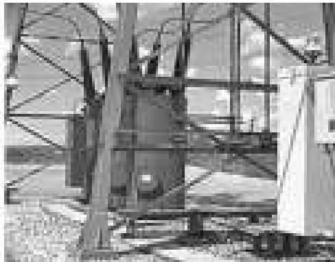
Oil Circuit Breakers in a Circuit
