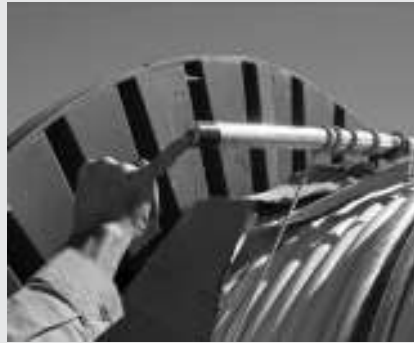
Figure 3 High-capacity low-sag conductor.
