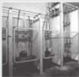
Figure 3 Air-insulated masonry cubicles
