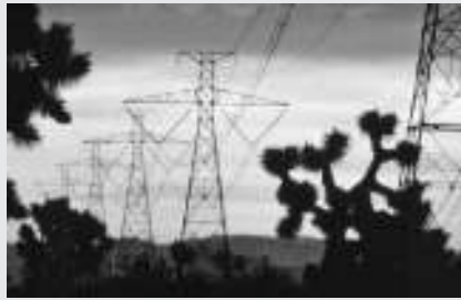
Figure 2 A \pm 500 -kV HVDC transmission line
