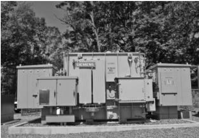
FIGURE 14.15 Three-phase 22.9 kVΔ/ 4.16 kVY distribution substation transformer rated 12 MVA OA/ 16 MVA FA1/20 MVA FA2. The transformer has fixed taps on the high-voltage side and an LTC on the low-voltage side (Courtesy of Danvers Electric.)
