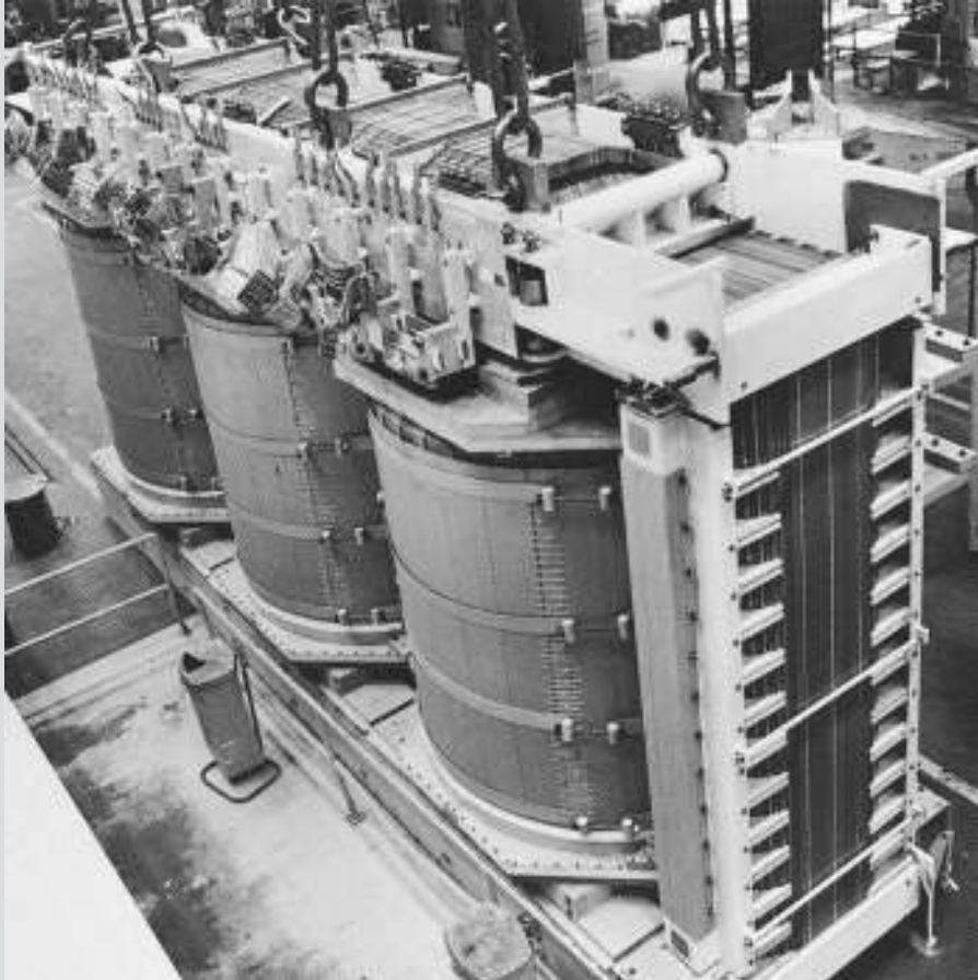
Core and coil assemblies of a three-phase 20.3 kVΔ/345kVY step-up transformer. This oil-immersed transformer is rated 325 MVA self-cooled (OA)/542 MVA forced oil, forced air-cooled (FOA)/607 MVA forced oil, forced air-cooled (FOA) (Courtesy of General Electric.)
