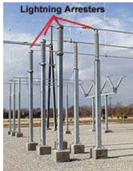
Lightning arresters on bus structures
