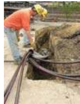
Underground transmission system.
