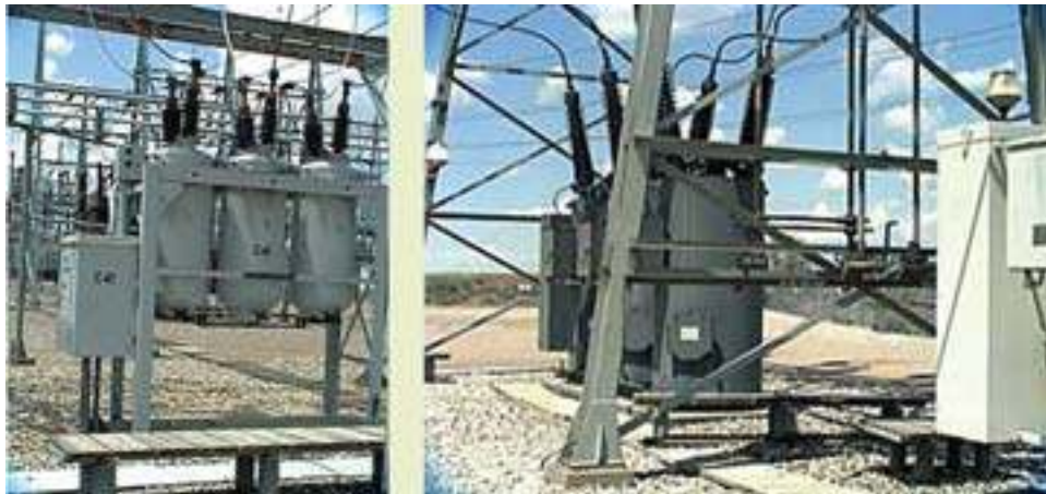
Oil Circuit Breakers
