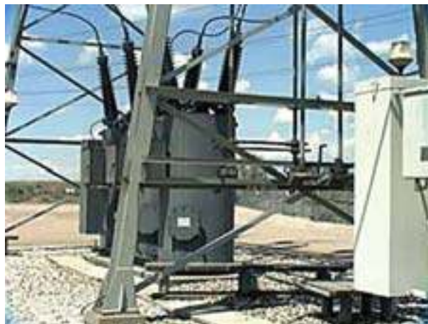
Oil circuit breaker
