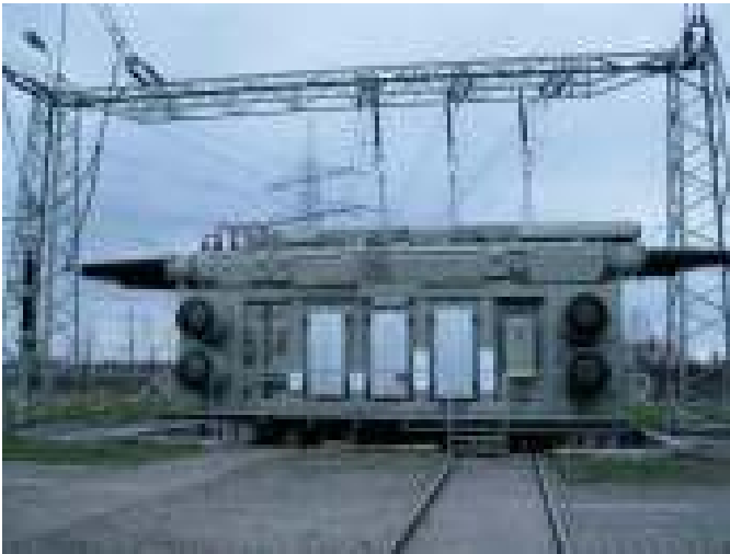
Figure 8.7 Overview of a transformer.
