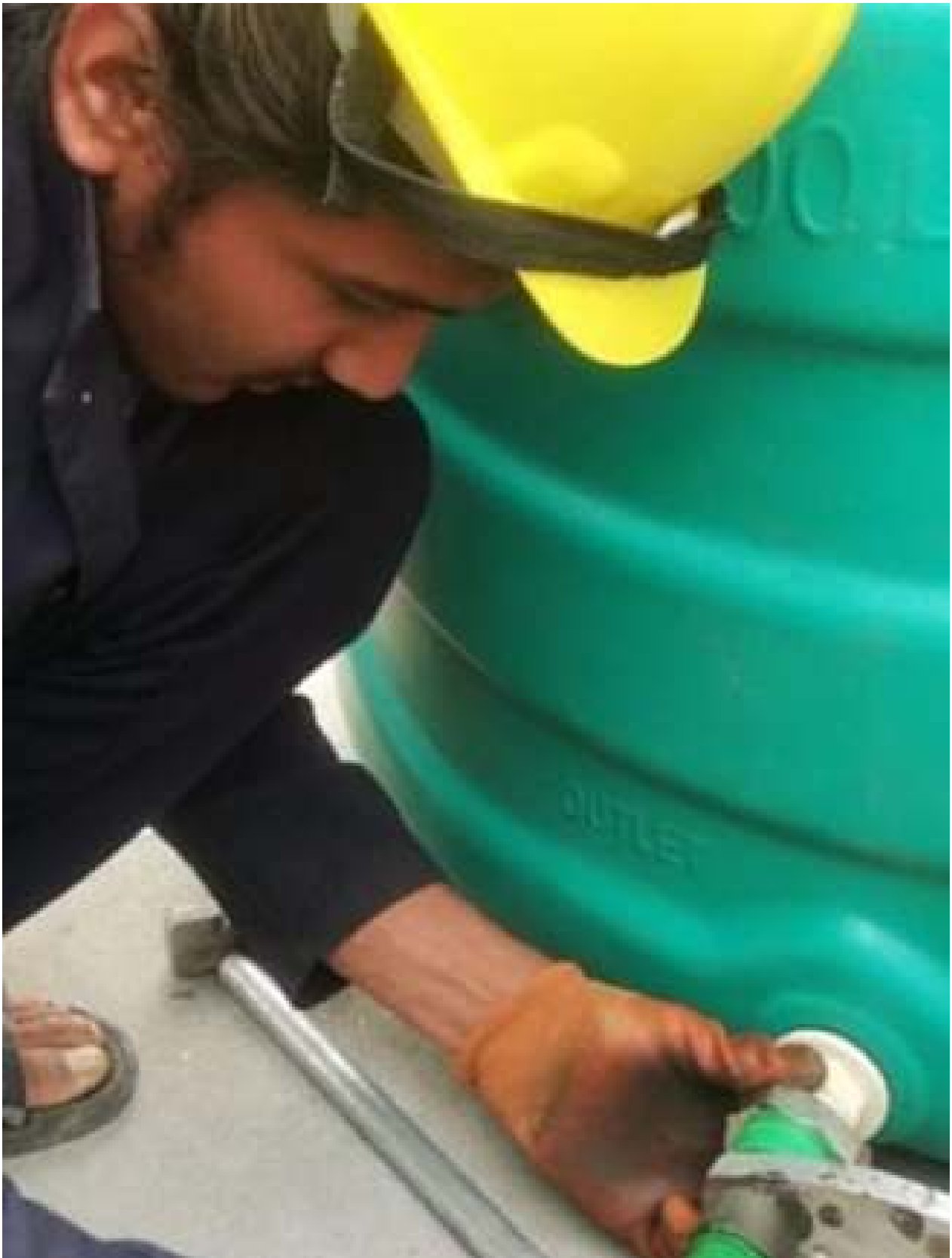
Pradip fits piping to a rooftop water tank. Soon, every home in his village will be linked with a municipal water supply through Nepal's One House, One Tap program, but for now, the homeowner who has hired Pradip will use a simpler gravity-based system for handwashing and toilet flushing.
