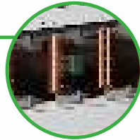
Main Busbar joint
