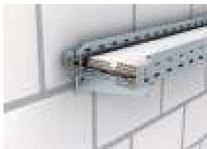
Reference laying type: E or F Cable on perforated cable tray, horizontal/vertical, e.g. type RKSM/MKSM
