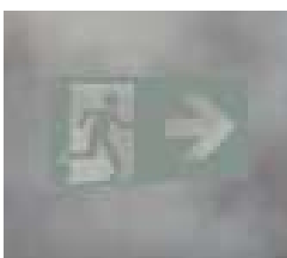
Badly illuminated escape sign
