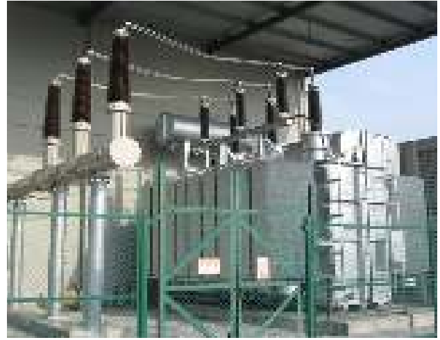
132/33kV 90/125MVA Power Transformer
