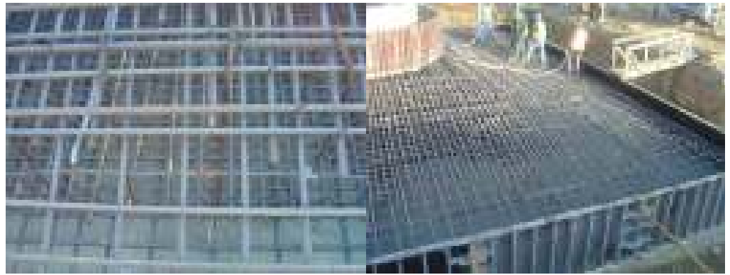
Image 13: Earthing system of a wind power plant
