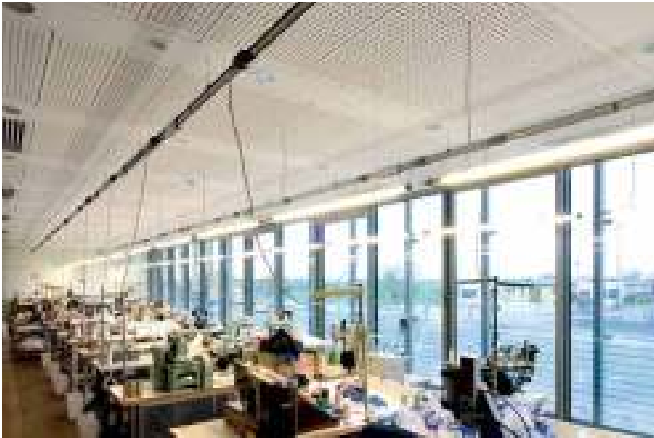
Example of lighting and small power distribution
