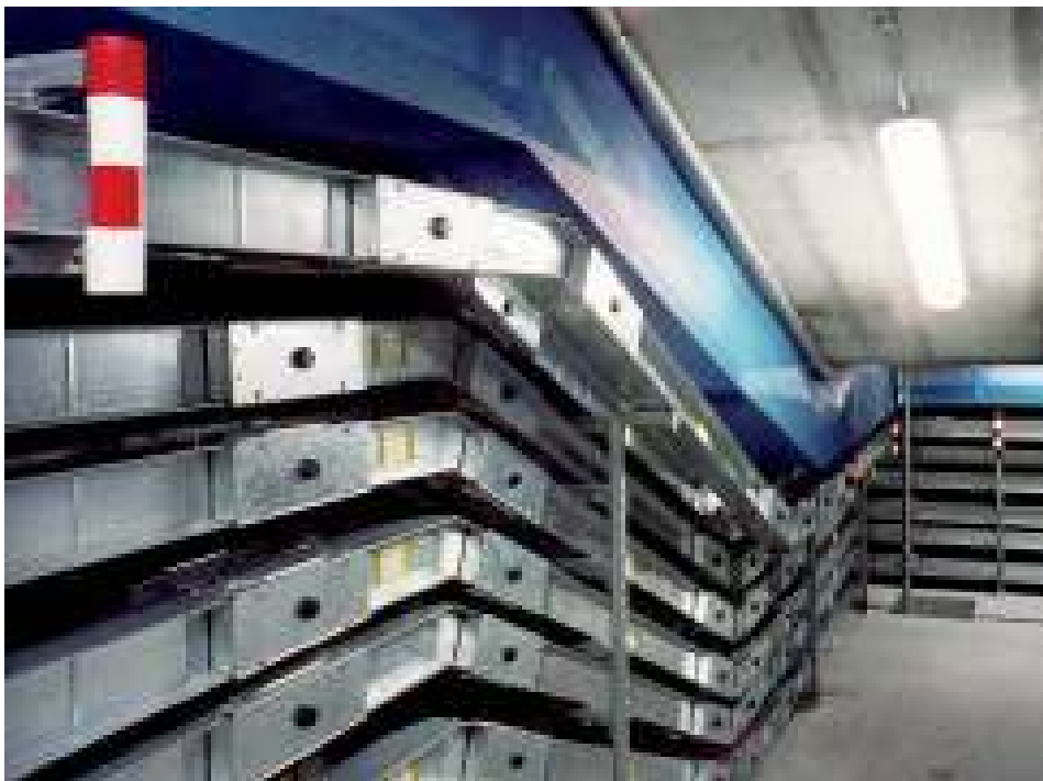
Example of high power distribution
