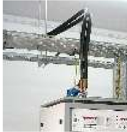
Figure 113. Incoming antenna circuits require protection.
