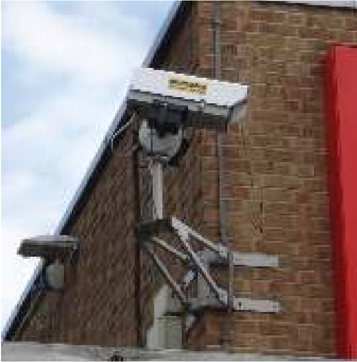
Figure 15. Violation of separation distance due to poor design and later additions to structure.
