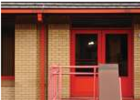
Figure 54. Example of poorly located adown-conductor.
