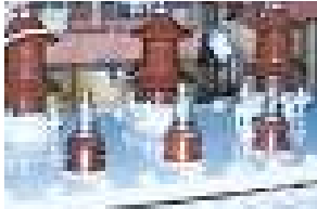
HV bushing with terminal connectors
