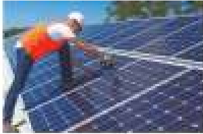
Requirements of the Solar industry
