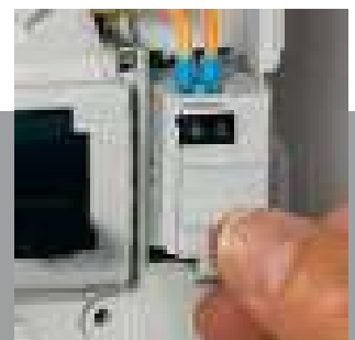
Auxiliaries are installed in dedicated locations under the front panel.
