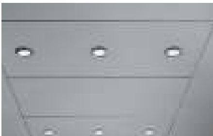
Ceiling lighting - standard LED round spot downlights
