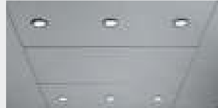
Ceiling lighting — Standard LED round spot downlights
