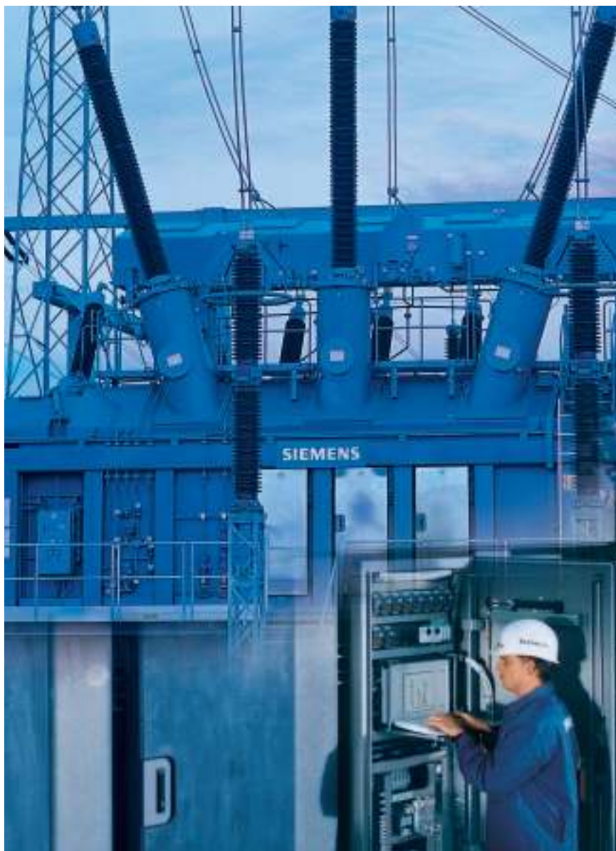
Fig. 45: An integrated solution – the complete Monitoring System housed in a cubicle of the transformer itself
