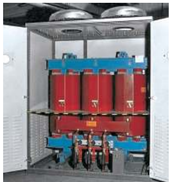
Fig. 54: GEAFOLE transformer in protective housing to IP 20/40
