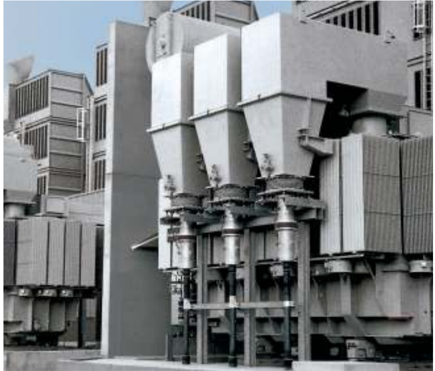
Fig. 14: Transformers with oil-filled HV cable boxes
